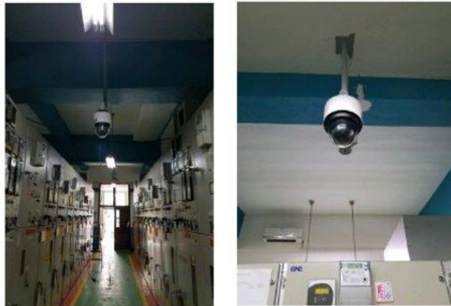
Ruang Kubikal 20 KV
