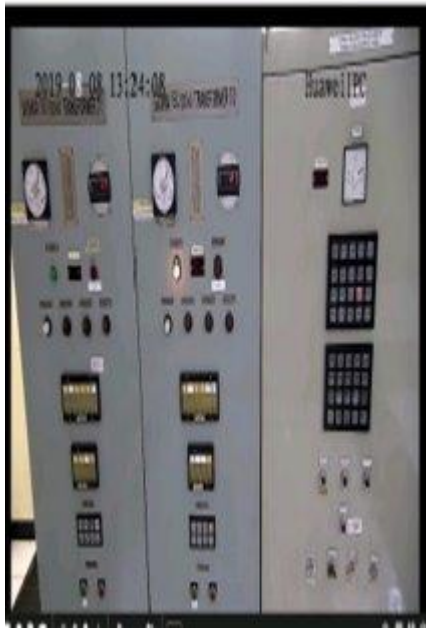
Ruang Panel Kontrol
