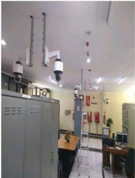
Ruang Panel Kontrol
